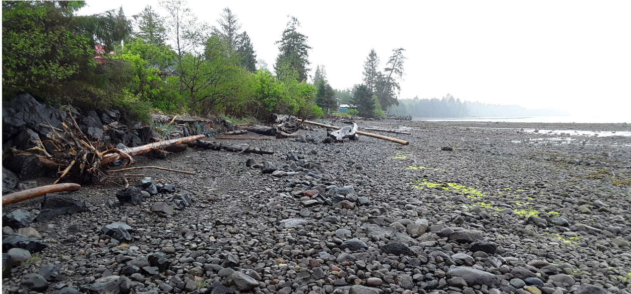
Figure 3-7. Erosion of the upper shoreline is evident in this photo, as are efforts to protect the shore with non-standard rock.
